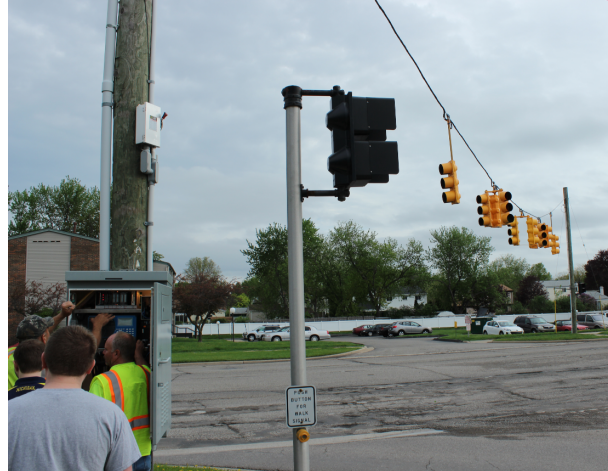
Figure 5: Intersection used for field tests. The targeted infrastructure controls a T intersection. The failsafe state of the intersection is a blinking yellow light on the main road and a blinking red light on the side road. At left is the traffic controller cabinet, which contains the controller, switch, and MMU. Radios and a video camera are located at the top of the pole.
